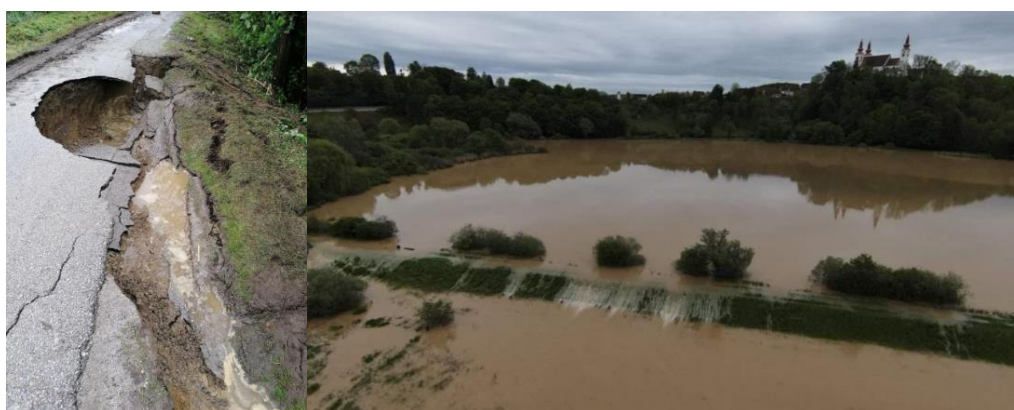
Fig. 5 Crest overtopping caused damage to the Gradišče dam
